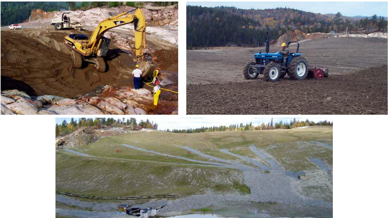
Figure 4 Photos showing cleaning of the pit perimeter prior to barrier layer construction (top left), cross-slope ripping of topsoil into the granular cover material (top right), and the finished pit cover in Sept-06 with the Collection Pond overshoot gate in the foreground (bottom)
